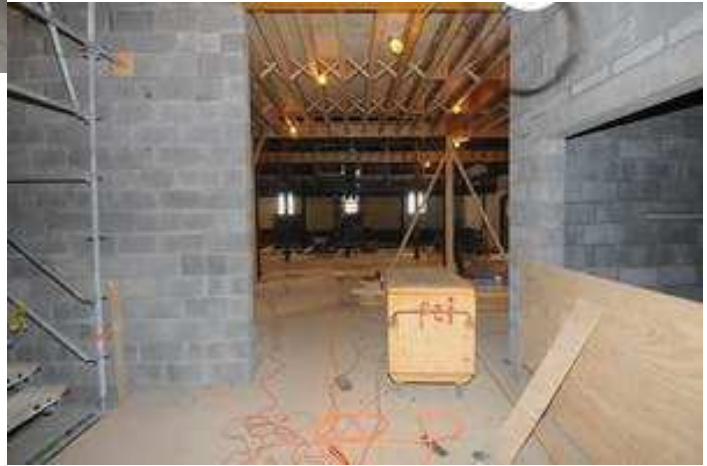
From the foyer: into the parish hall with stairs to 2nd floor on the left and the new 2nd flooring in place
