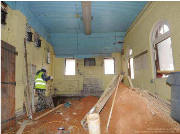
The kitchen is prepped for its new floor and walls to support the new clergy offices above.
